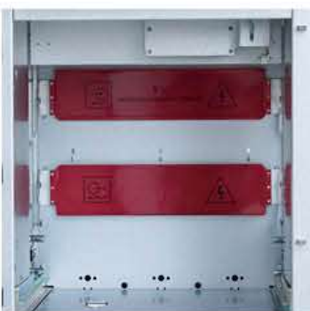
Circuit breaker room
