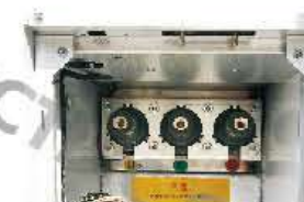
Cable connection room
