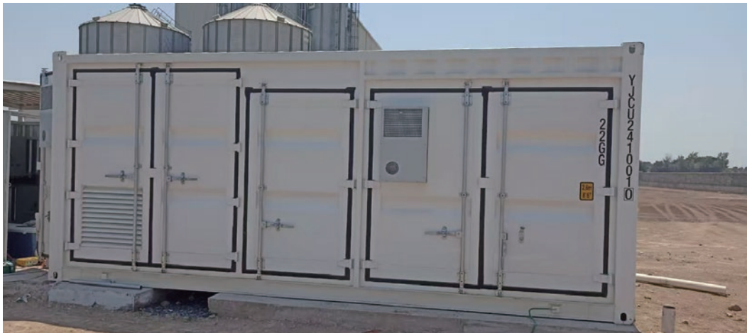
Mexico 500KW 1MWH integrated BESS
