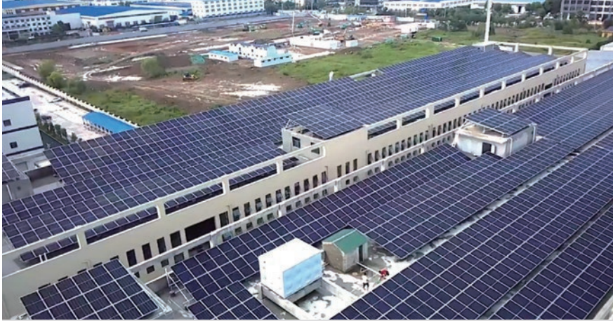
1.88MW Roof Solar System
