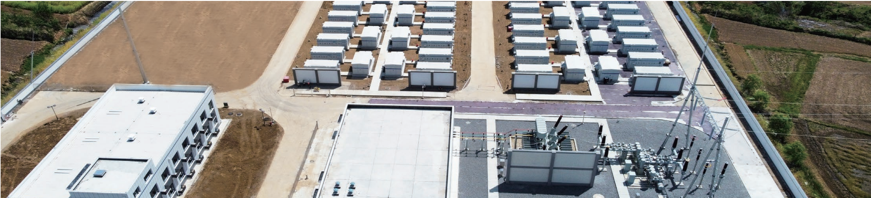
200MW/400MWh Battery Energy Storage Project
