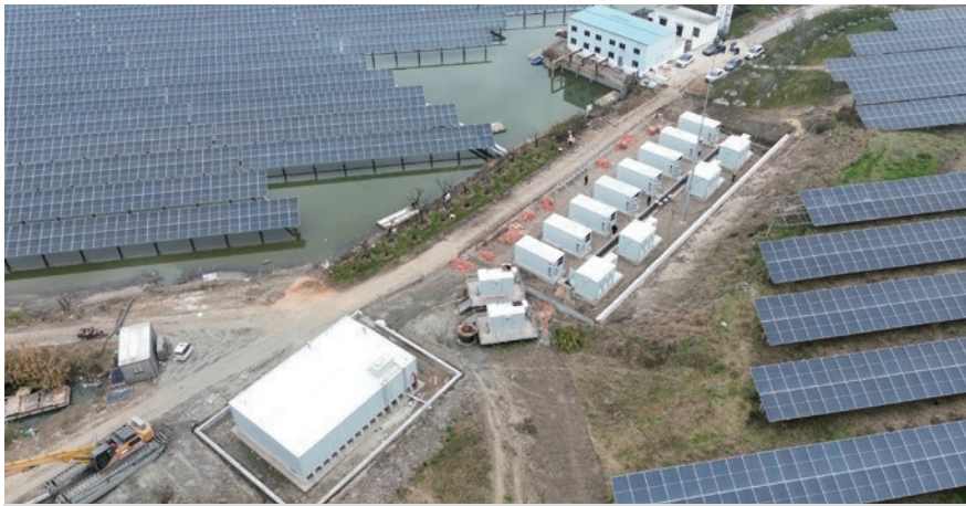
20MW Solar Plant+40MWH BESS
