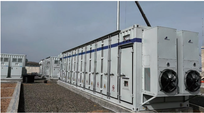
100MW Solar Plant + 40MWH BESS
